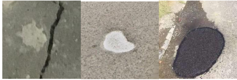
Fig. 1: (a) crack, (b) pothole, (c) patch.
